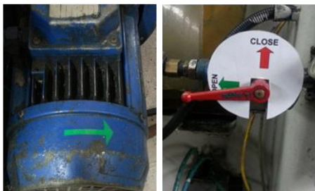
Figure 1: Directional flow markings added to motors and valves
